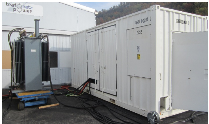
Our LFH plant connected to a 2 MVA transformer
