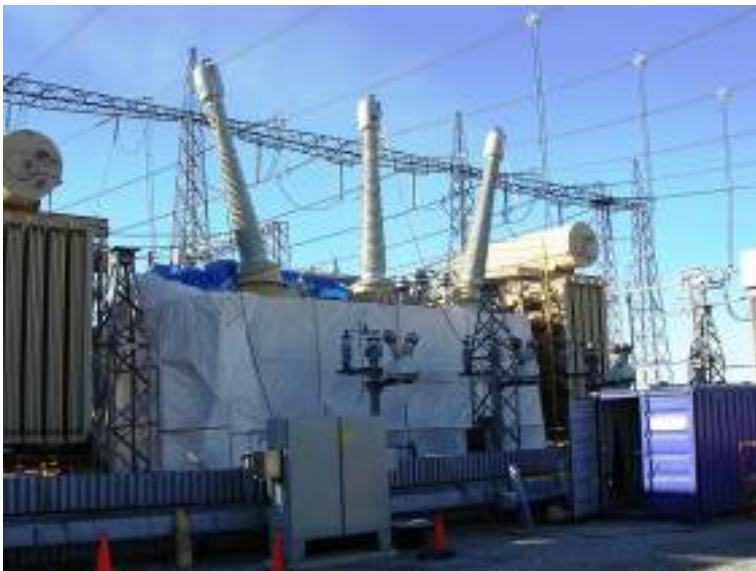
LFH drying of a 750MVA/500 kV autotransformer (picture: ABB)
